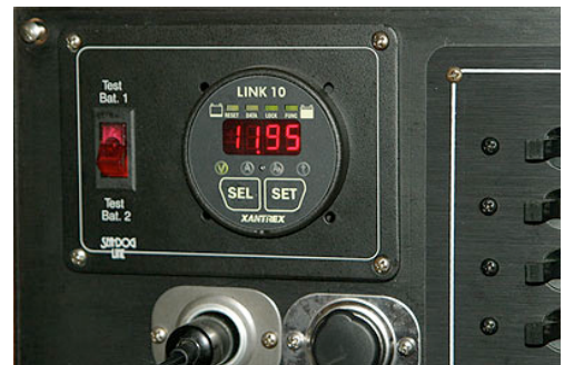
Amanzi's Voltmeter / Amppmeter. It tells us the charge on our battery bank & how much power we're using or charging at any given time
